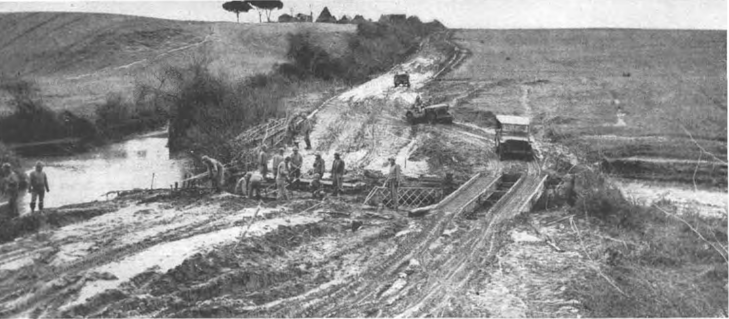
ENGINEERS BRIDGE A STREAM on a road from Nettuno to the front. Frequent rains and enemy shell-fire damage made this a difficult task, but the roads had to be kept open to move armor against the Germans.
