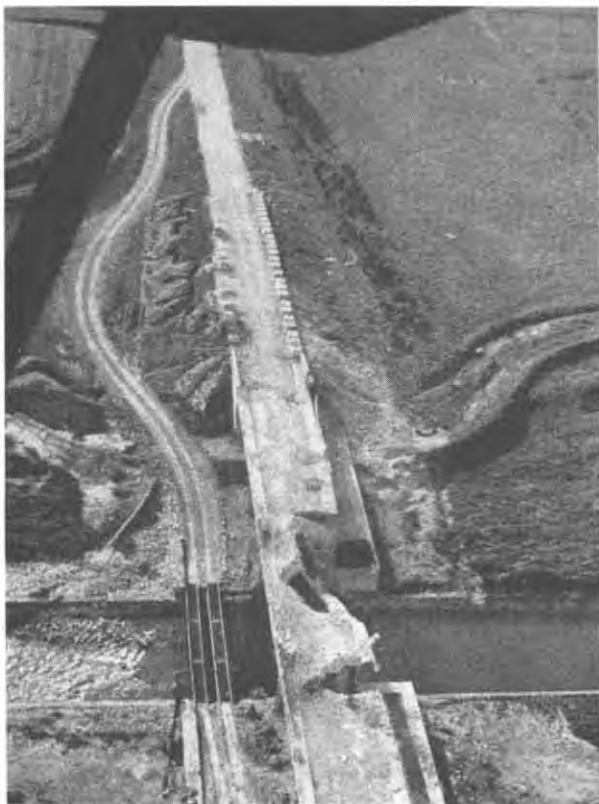
A DESTROYED MUSSOLINI CANAL BRIDGE near Borgo Sabotino, part of the reconnaissance effort on the right flank on D Day. Photo, taken later, shows a tread-way bridge over the canal, concrete road blocks (German) on the far side, and a trench system dug by American forces.
